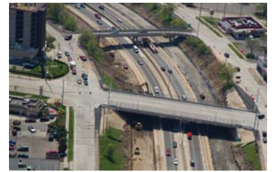
Incentives were offered to shorten the amount of time the bridge would be closed.
